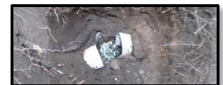
Broken septic pipe from a home in Gratiot County; found & repaired with the help of Mikie V. and Akers Waste Removal.
