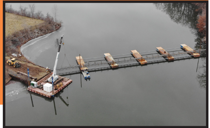
Temporary bridge being constructed across the Pine River to support system utilities and piping. See page 1 for updates on the Velsicol Burn Pit work.
